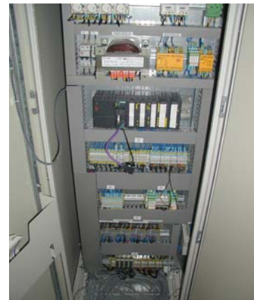
Besturing (PLC Siemens S7)
